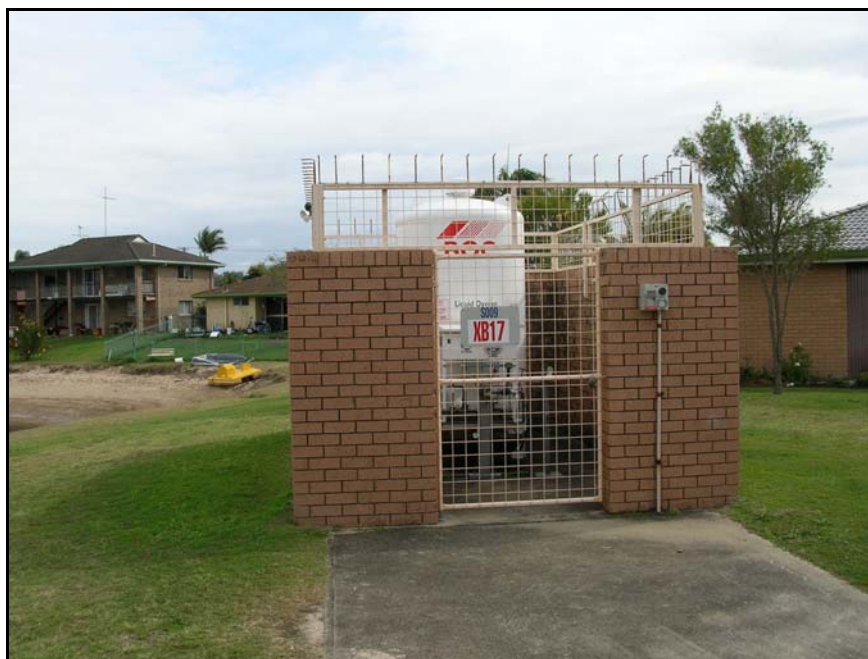
Figure 3 An oxygen injection station
